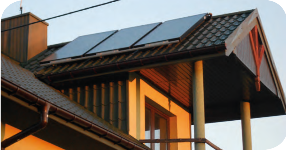
Solar installations on the roof in city of Myszków Copyright: city of Myszków
